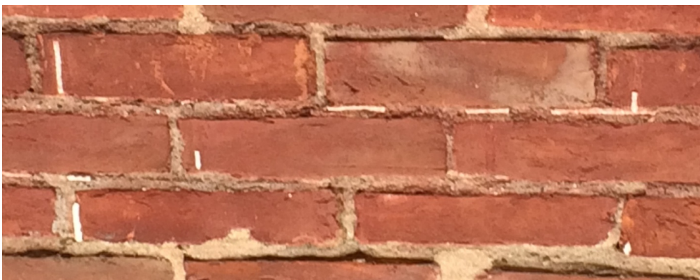
Remnants of Lined Mortar Joints, detail of David Hawes House
